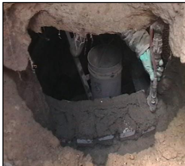
Before- force main destroys MH wall.
